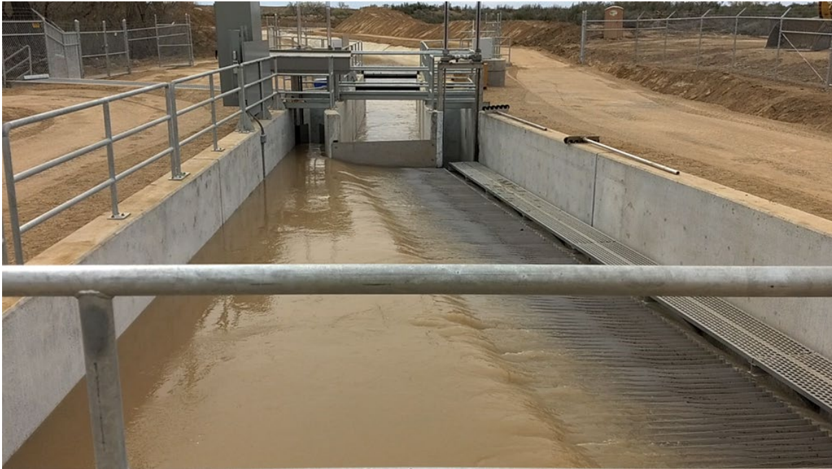
Figure 1. Green River Canal fish screen in operation, looking downstream. Water flows left to right over the screen (foreground right). Screened water drops into the canal entrance while fish and unscreened water is collected and diverted back to the Green River. Note the gap above downstream end of screen, which could allow jumping fish a means enter the canal. Photo: Ryan Christianson
