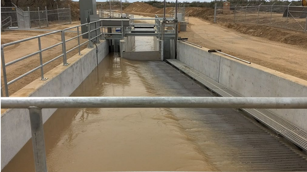
Figure 1. Green River Canal fish screen in operation, looking downstream. Water flows left to right over the screen (foreground right). Screened water drops into the canal entrance while fish and unscreened water is collected and diverted back to the Green River. Note the gap above downstream end of screen, which could allow jumping fish a means enter the canal. Photo: Ryan Christianson, USBR.
