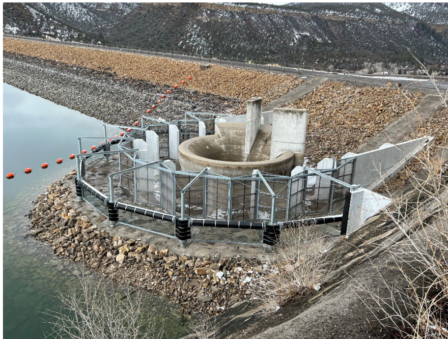
Photo 10. Fish screen to keep fish inside Ridgway Reservoir, Ridgway Colorado. Photo credit Kyle Kissner, Kissner General Construction
